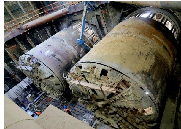
LAMTA Purple Line Sections 2 & 3 Tunnels, Stations, & Systems Los Angeles, CA PROJECT VALUE: $3.82B
