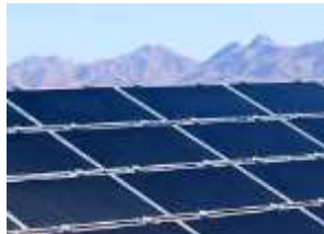
Yuma Foothills Solar 35 MW
