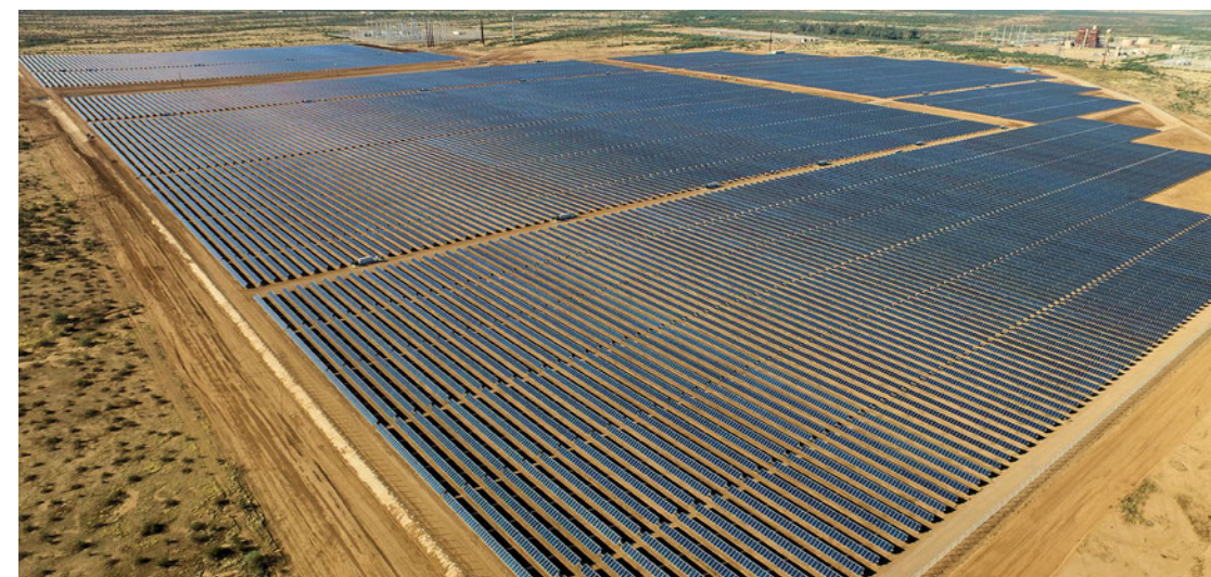
Red Rock Solar Plant — located south of Casa Grande, Arizona and completed in 2016.
