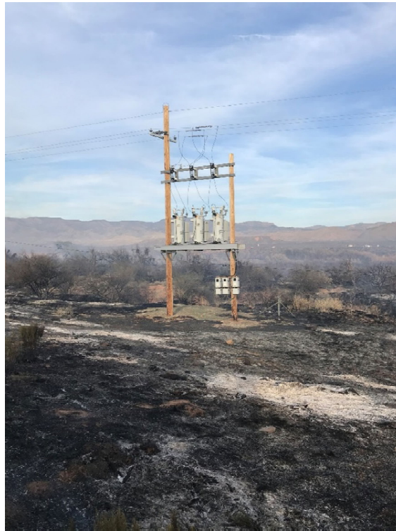
Figure 5. Defensible Space Around Equipment that was Protected in Extreme Fire Conditions
