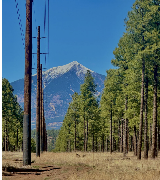
3 Figure 10. Wooden Poles Wrapped in Fire Mesh
