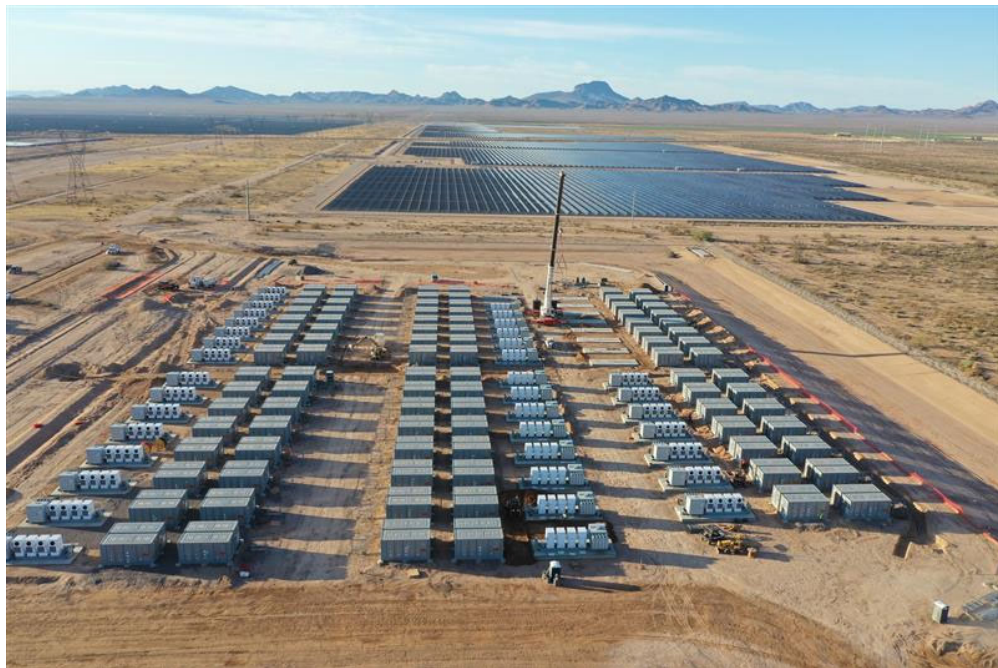
Figure 11. Agave BESS Storage
