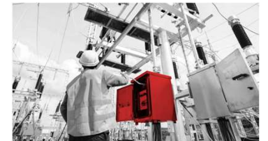
Enclosures Control Panels
