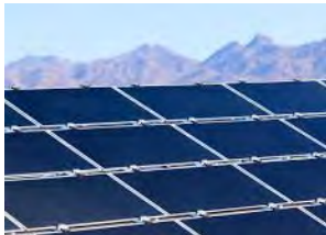
Yuma Foothills Solar 35 MW
